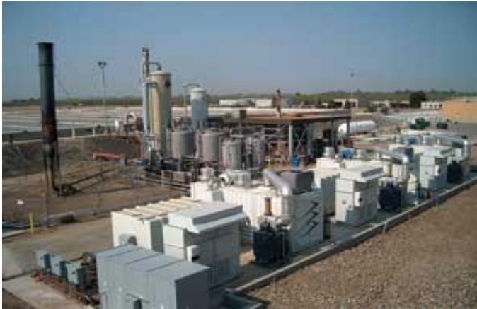
Original Installation of Three FuelCell Energy Fuel Cells and Gas Pretreatment Unit at Tulare Wastewater Treatment Plant.
