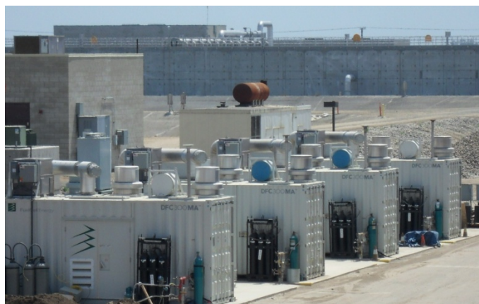
Four FuelCell Energy Fuel Cells at Tulare Wastewater Treatment Plant. Photo courtesy of Tulare Wastewater Treatment Plant.
