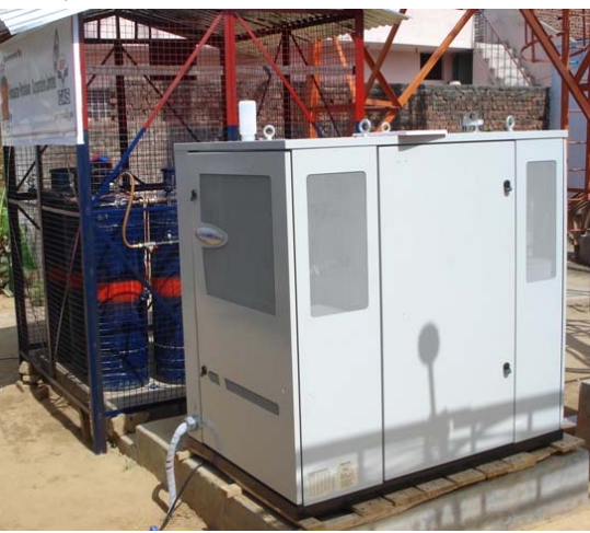
Plug Power GenSys system in India
