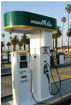
Riverside Hydrogen station
