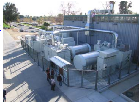
1-MW FuelCell Energy fuel cell
