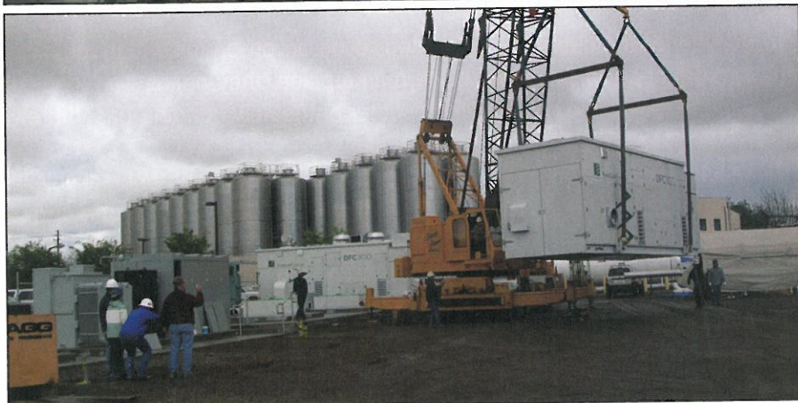
TOP: A schematic of UTC fuel cell. This similar to the type installed by Sierra Nevada Brewing Co. of Chico, California. CENTER: Sierra Nevada's four FuelCell Energy 250kW DFC 300 fuel cells. BOTTOM PHOTO: Installation of fuel cell plant underway at Sierra Nevada.
